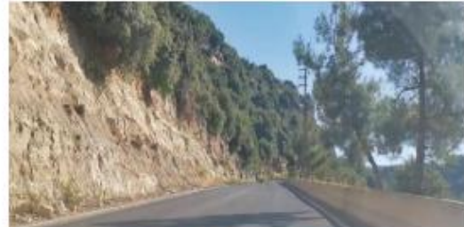
No berm, no slope protection
