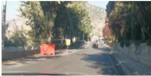
Failed retaining wall
