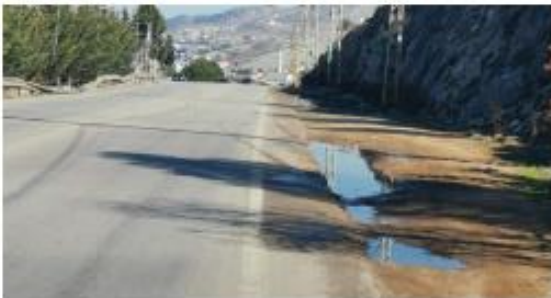
Drainage problem and damaged guardrails
