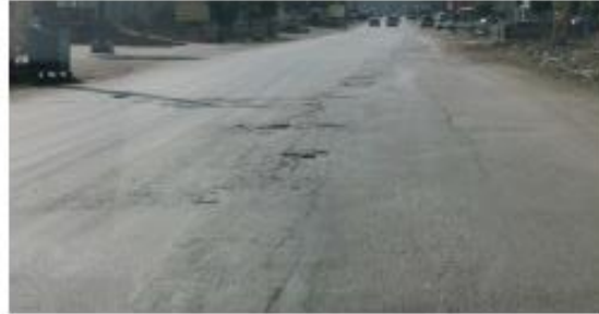
Deep pavement damage due to water infiltration
