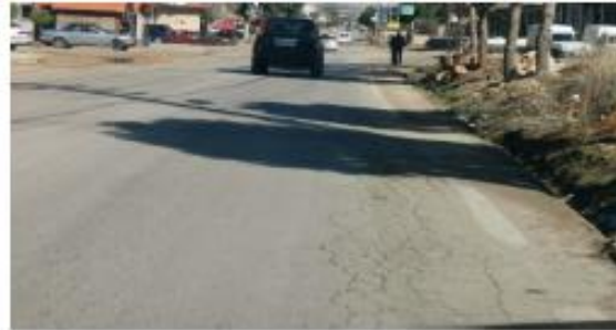
Bad earth ditch causing failure to the asphalt
