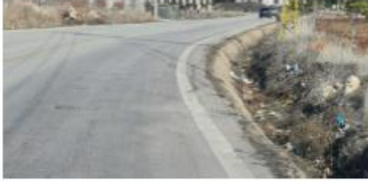
Obstructed channel presenting high risk in its shape to the road users
