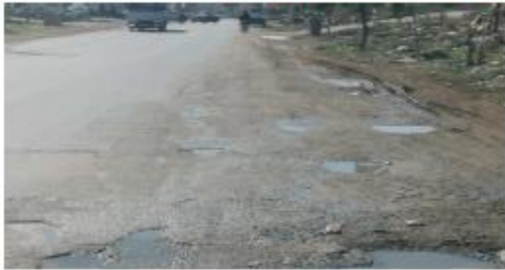
Deep pavement damage due to water infiltration
