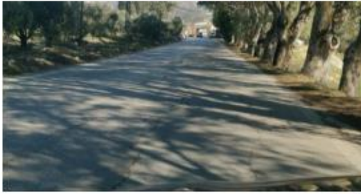
Damaged pavement due to absence of drainage
