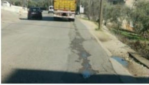
Main problem is stagnant water No Safety barriers
