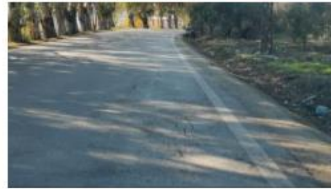
Obstructed channels and damaged pavement
