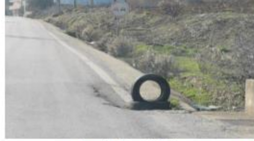
Depression due to water infiltration
