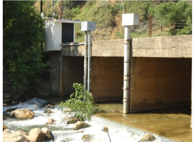
Equipments of the Marj Bisri Station : Limnigraph, Rain Gauge and Anemometer
