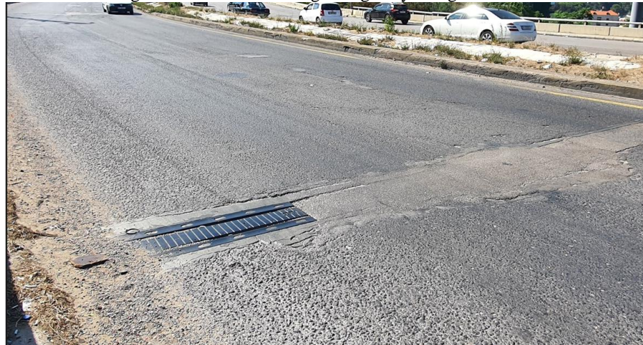
Photo 1 - Existing condition of one damaged Highway Bridge Joint
